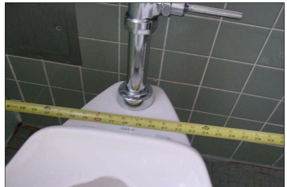
Girls Restroom Across from Room 25 Admin. Building
