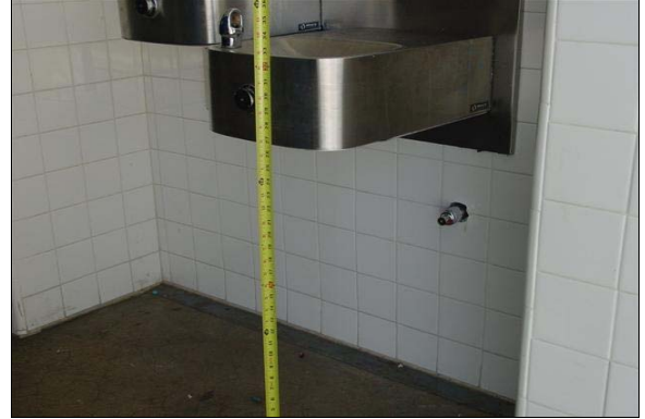
Drinking Fountain Second floor Administration Building
