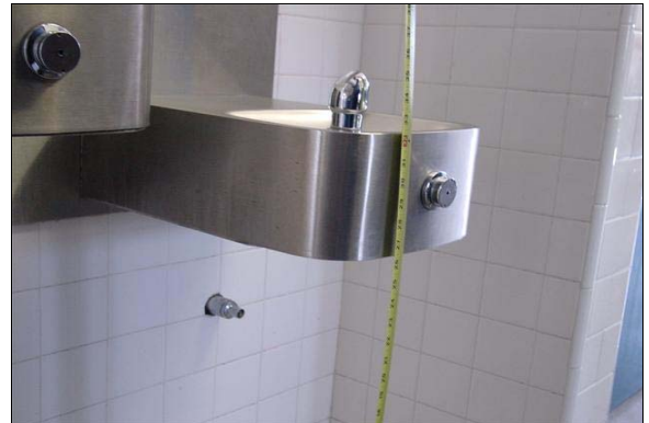
Drinking Fountain Second floor Home Economics Building
