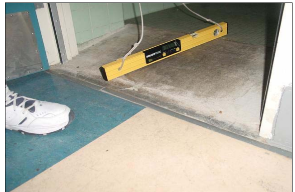
Girls Restroom Across from Room 25 Admin. Building
