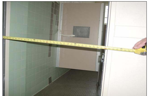
Girls Restroom Across from Room 25 Admin. Building
