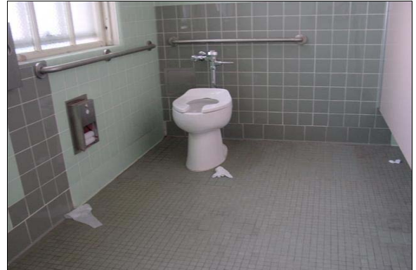
Girls Restroom Across from Room 25 Admin. Building
