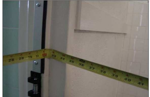
Girls Restroom Across from Room 25 Admin. Building
