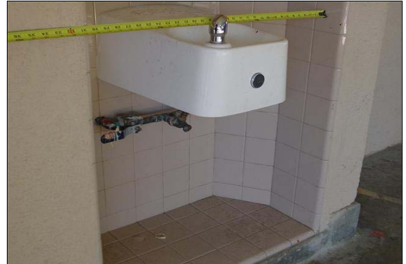
Drinking Fountain Next to the Administration Office
