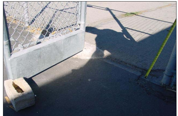
Gate to Accessible Parking Next to Room B6
