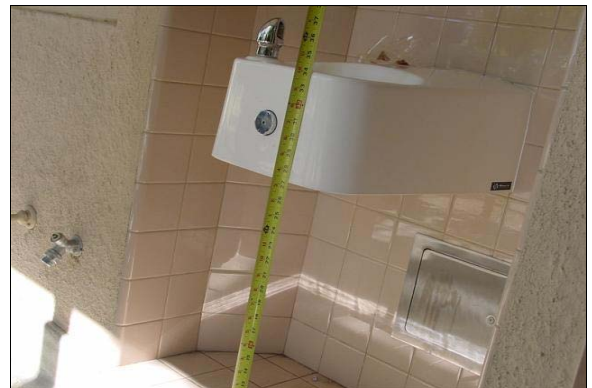
Drinking Fountain Next to Room 42A
